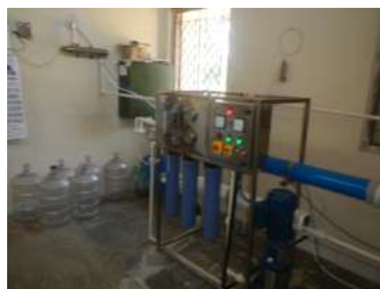
R.O. Unit facility
