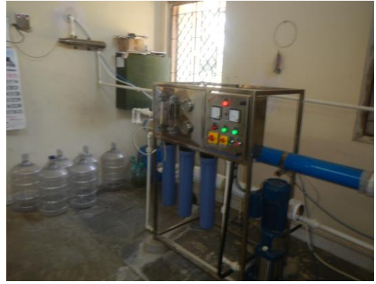
R.O. Unit facility
