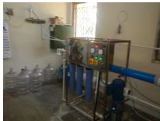
R.O. Unit facility
